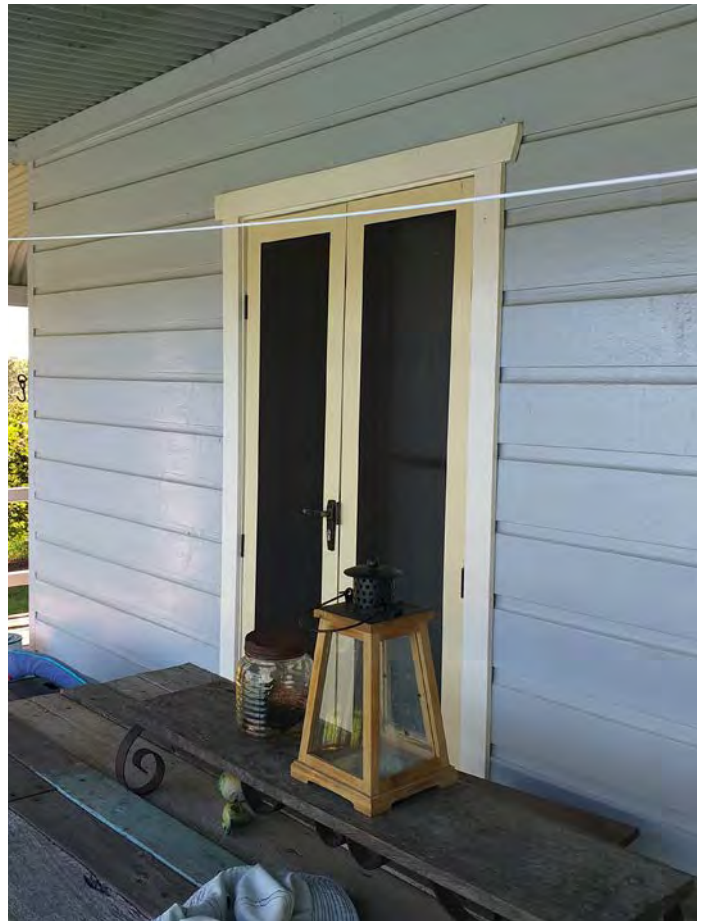
Figure 60: Rusticated timber weatherboard cladding. Eight inch boards were used to clad the exterior while five inch boards are used for interior linings. Source: TZG Heritage, 2024.
